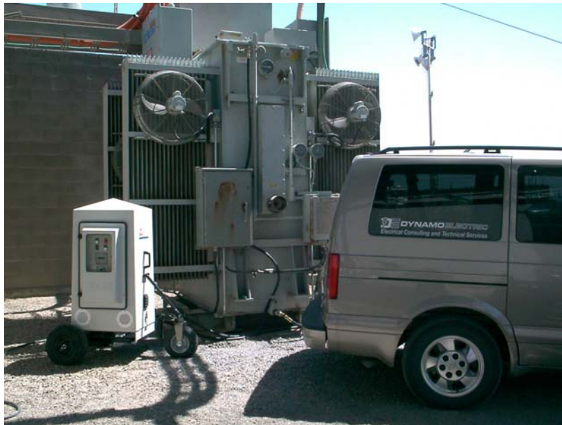
In this case the V30 CJC Vacuum Filter on-line transformer oil processing unit is being used to add top-up oil and remove moisture from a 6 MVA transformer.
